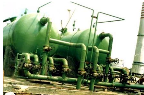
At site as Installed
